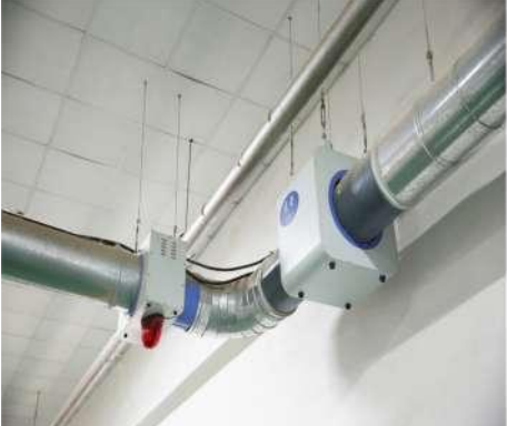
MULTY DUST FILTRING UNIT
